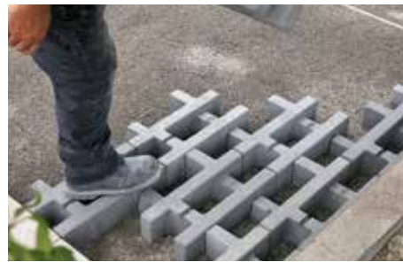
Boulevard Verde pavers are laid in strips on a conventional densified granular foundation.
